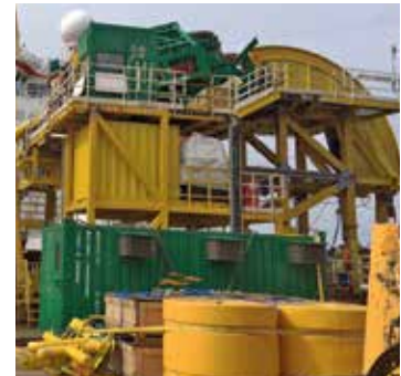
Electrical power unit and control cabin
