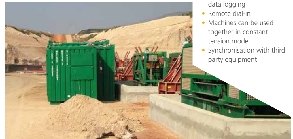
Power unit container.
