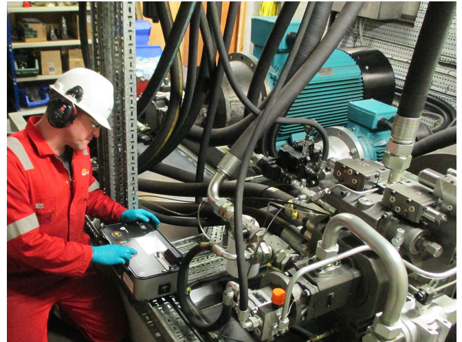
On-site technician carrying out hydraulic system checks
