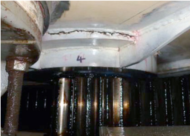
Initially identified floor cracks
